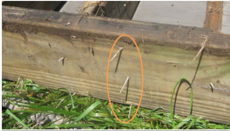
Photo: A nailed-only deck ledger connection is dangerous.
