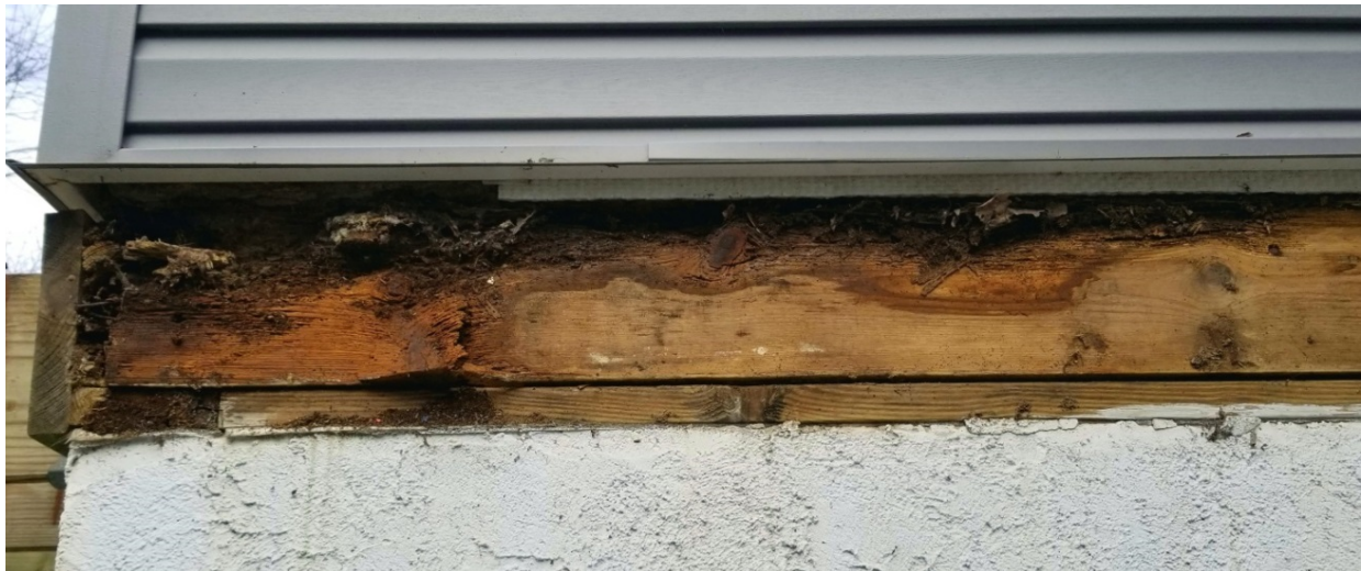
Photo: House band joist with no house wrap or flashing behind the deck ledger
