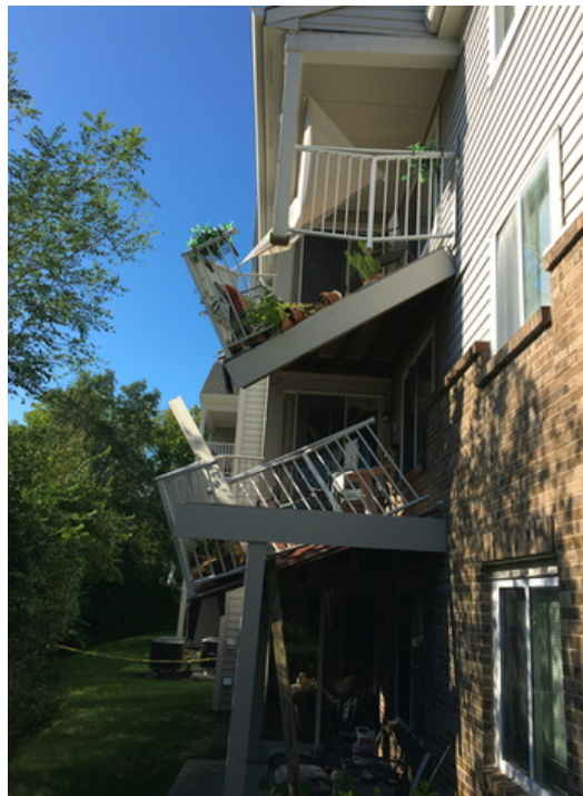
Photo: 2018 Balcony Collapse Courtesy WCPO-TV
