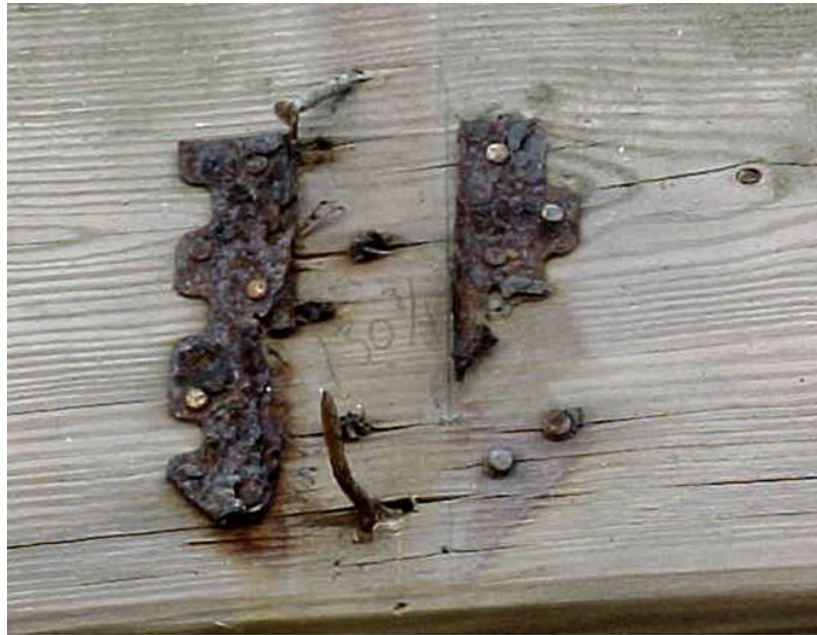
Photo: Coastal joist hanger after wedding party deck collapse
